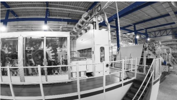
Proven technology: CP line running at full capacity
