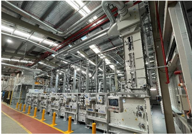
ANDRITZ reXline tearing for textile recycling at Sealy Australia's mattress plant in Brisbane
