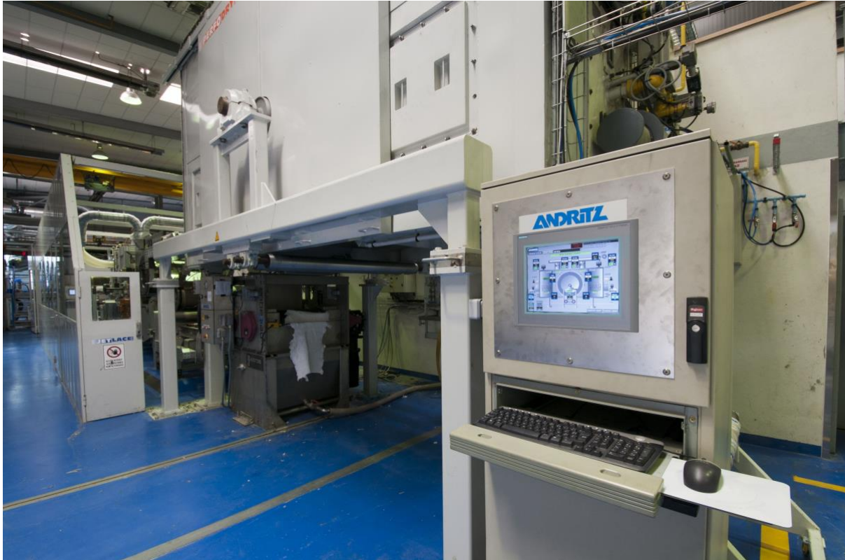
Spunlace pilot line at ANDRITZ Perfojet, France
